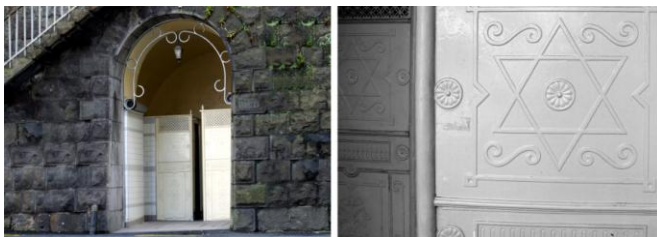
Figure 3: Cast iron screens at the entrance to The Star of David. Durham Street West. Auckland 1880.
