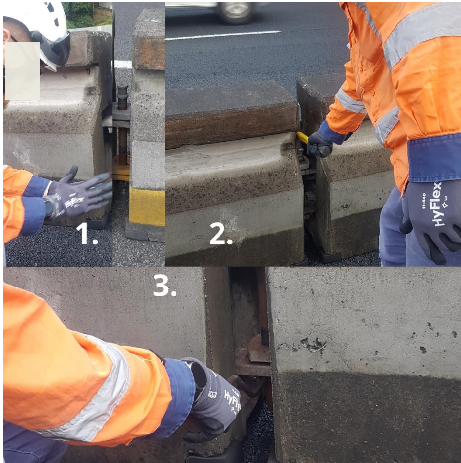
Fig. 5: Manual Pin inspection by NZTA staff. 1. Unsafe pin found during the manual inspection, 2. hammering down the metal pin, 3. securing the safety latch.
