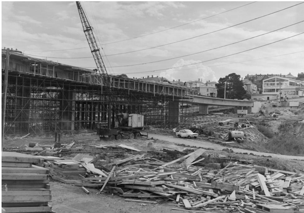
Figure 26 Newton Road ( Donovan, 1973 ). Image of the construction waste from the demolition of residential housing across the site and the redevelopment of Newton Road as an overpass for the Motorway Junction.
