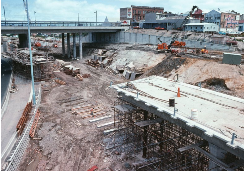
Figure 27 Looking south from Hopetoun Street toward Karangahape Road ( Donovan, 1975). Image showing the construction of motorway ramps and road embankments.
