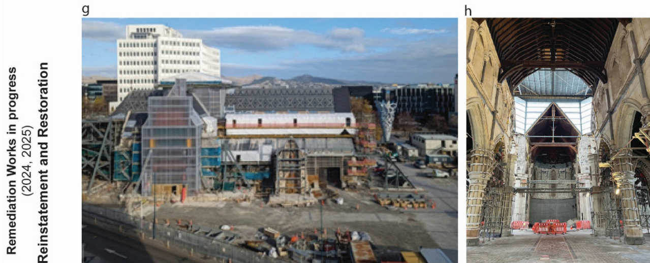
Figure 5. Post-earthquake damage, interventions, and remediation, Christ Church Cathedral. (a) Post-earthquake damage, seen from Cathedral Square, 2011. Photograph by Jason Ingham. (b) Post-earthquake damage to Cathedral tower, 2011, seen from Cathedral Square. Photograph by Jason Ingham. (c) Post-earthquake collapse of Cathedral tower and damage to primary façade 2011, seen from Cathedral Square. Photograph by Jason Ingham. (d) Emergency stabilisation for primary façade, 2015. Photograph by Jason Ingham. (e) Stabilisation works underway, 2021. Photograph by Jason Ingham. (f) Post-earthquake securing for primary façade, 2021. Photograph by Jason Ingham. (g) Post-earthquake external remediation works, 2024. Photograph by Stacy Vallis. (h) Post-earthquake internal remediation works, 2025. Photograph by Julia Gatley.
