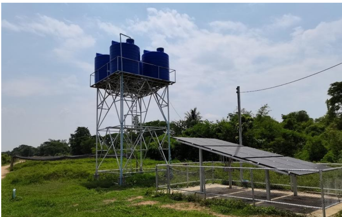
Figure 10: Solar Panels in BMM5
