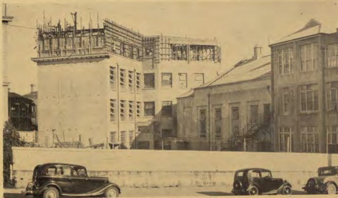
A view of the partially completed storey on top of the workshop block.
