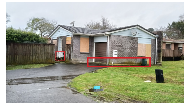
5. House with low floor level; Elevation of door is not high enough; The air condition unit is placed on ground level.
