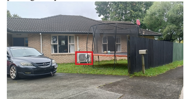
6. The air condition unit is placed on ground level.
