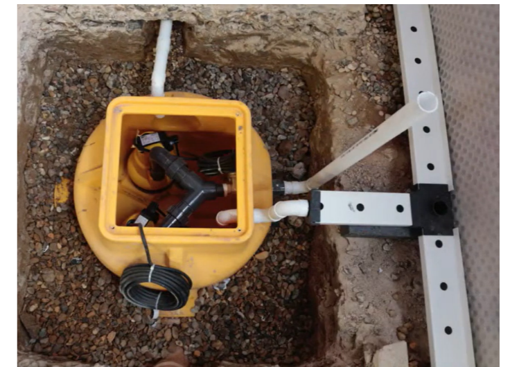
Below: Figure 7.21 An automatic 'sump pump' connected to drains in the floor (BRE Group, 2017)
