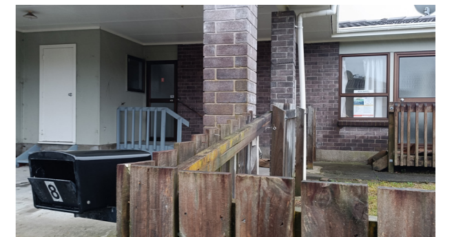
14. This house was damaged in the flood, resulting in material leaks and mould growth; it is currently under access restrictions and vacant.
