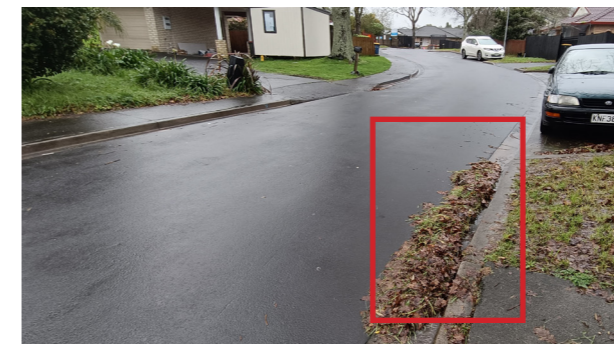
13. The ditch was blocked by fallen leaves and grass clippings.
