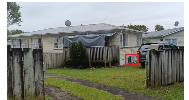
8. The air condition unit is placed on ground level.
