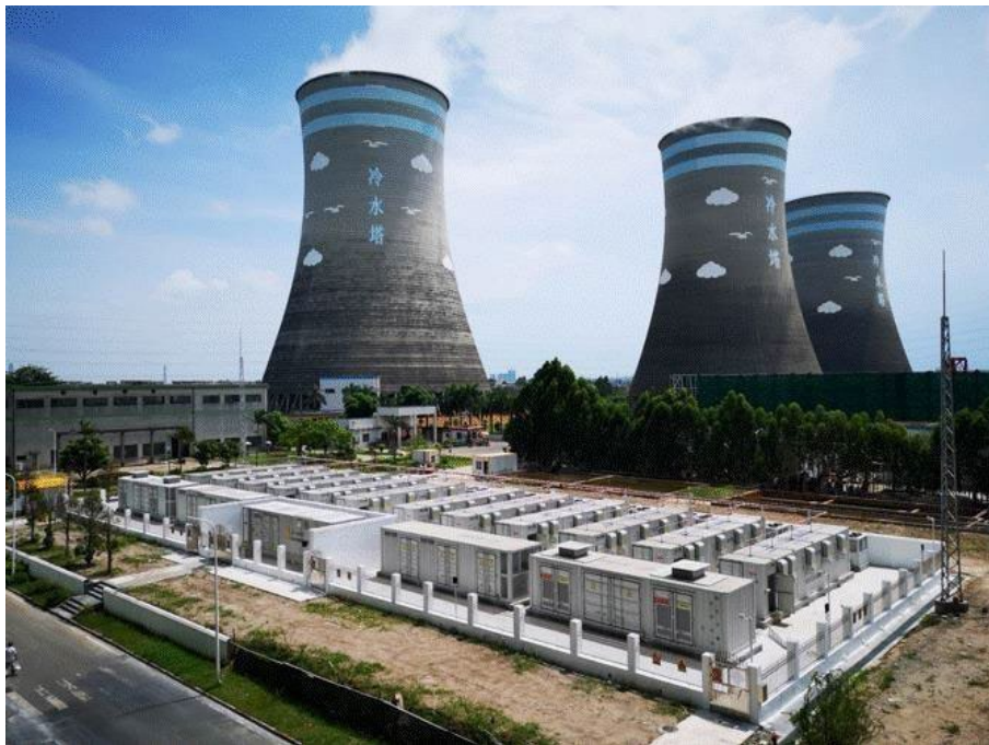
Figure 1.1 Construction of a 20MW/10MWh BESS at a 600MW coal-fired power plant to improve frequency regulation quality.
