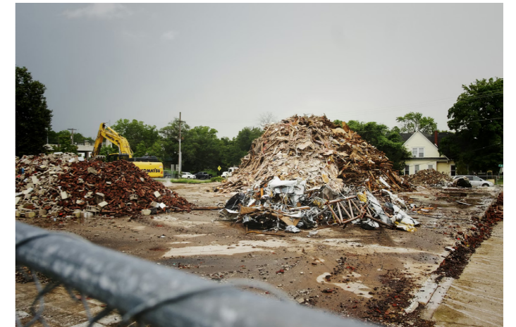
Figure 2. A Pile of Debris on the Side of a Road
