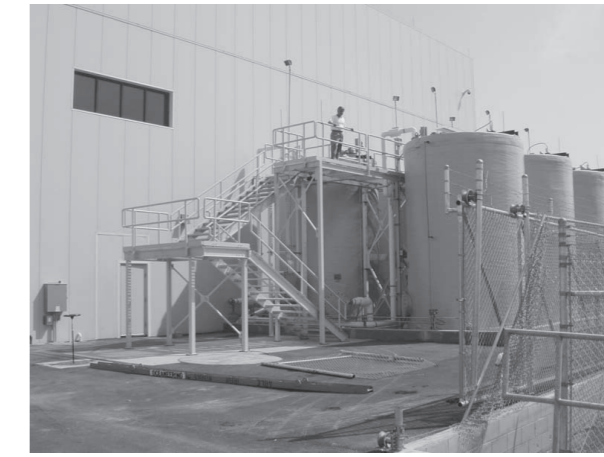
Figure 34: Six Mixing Tanks Located Outside the Building (Michael, 2004, p142)
