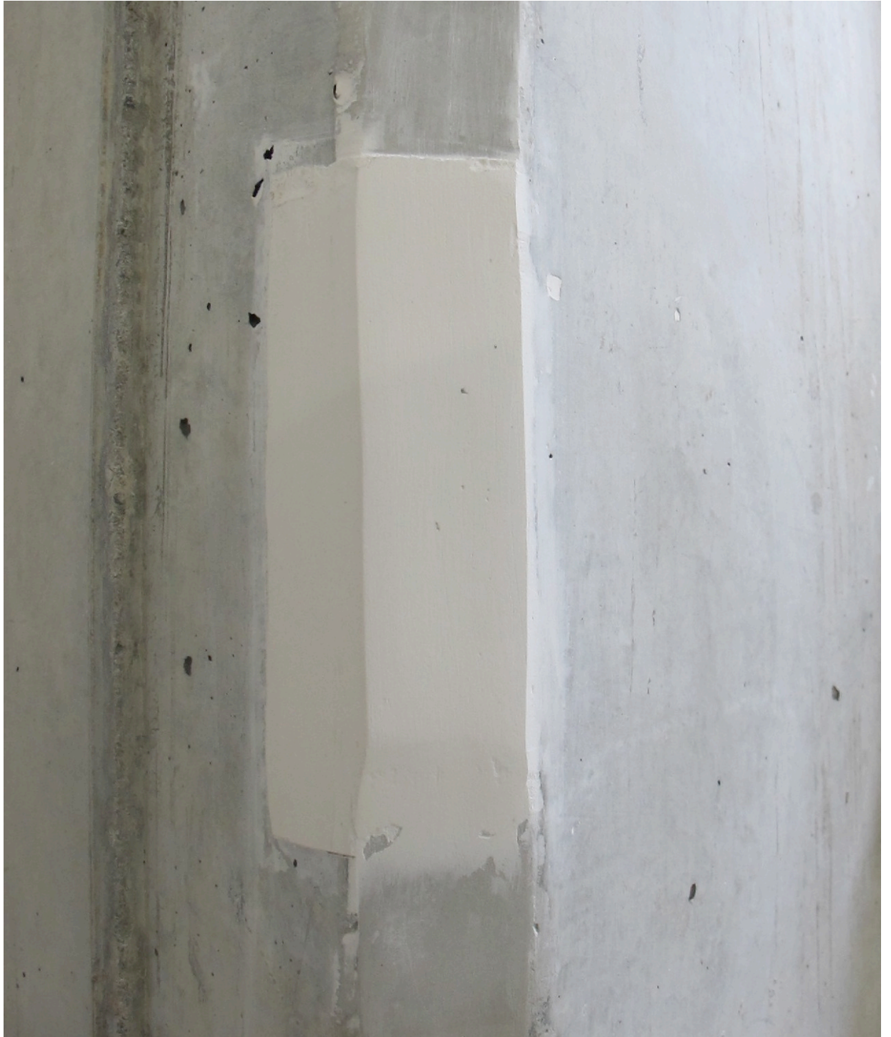
Subject[ed] Matter , Installation detail, Gib Stopping Plaster (applied Directly to concrete wall), AUT, 2013
