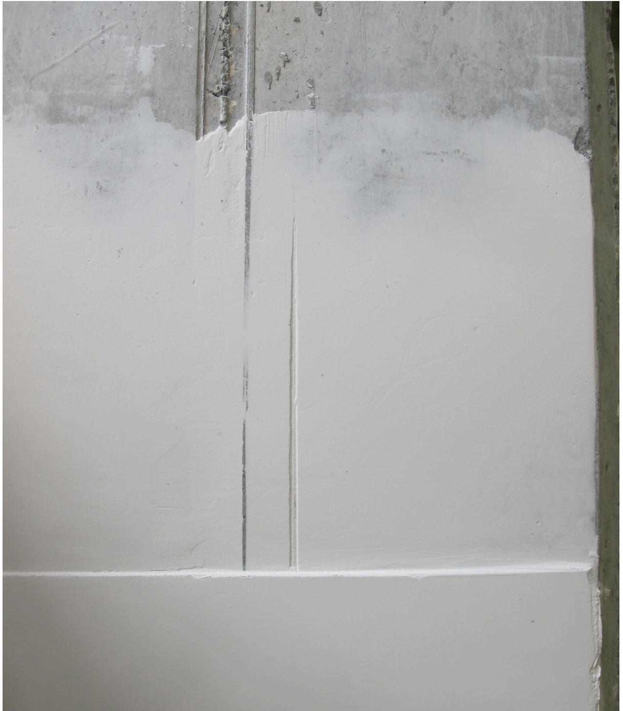
Subject[ed] Matter , Installation detail, Gib Stopping Plaster (applied Directly to concrete wall), AUT, 2013
