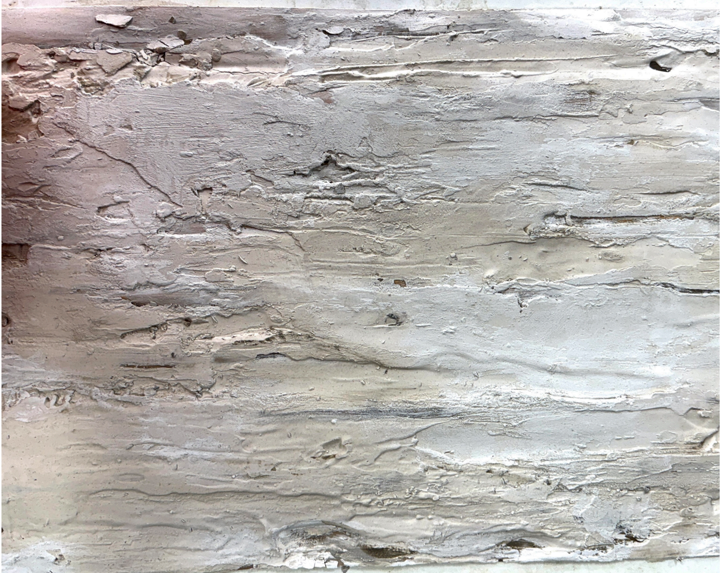
Figure 42. M Refiti. Chipped Plaster , CE-1 - Cracked Plaster Surfaces, 2024, Photography.
