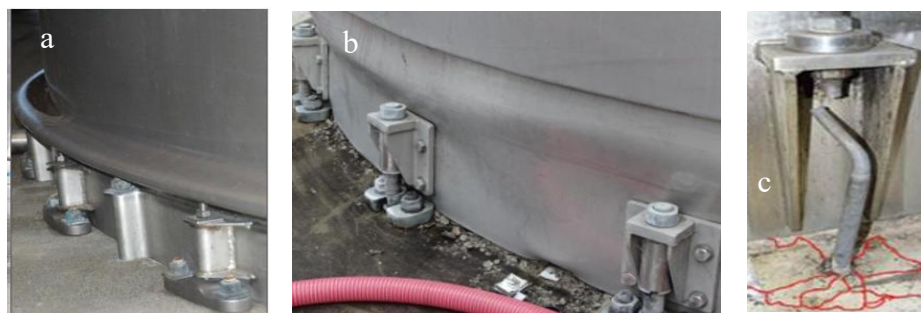
Figure 7-4: Reported damage in Kaikoura earthquake; (a,b) Barrel buckling; (c) Rod rupture [14]
