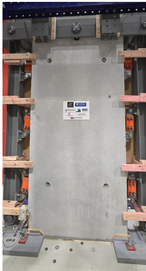
Figure 5-28: Post-Test Condition: Left-Side Joints Ruptured, Right-Side Joints Intact
