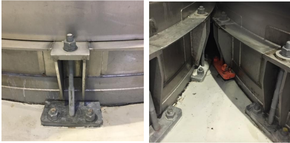
Figure 6-8: Example of existing tank connections
