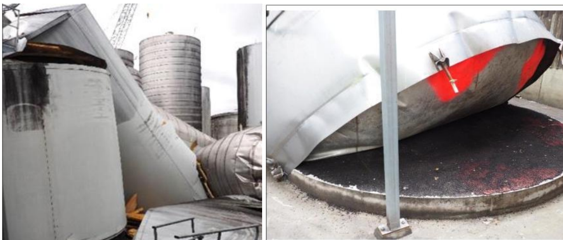
Figure 2-33: Complete collapse of different sized tanks (Dizhur et al., 2017 and Fischer et al., 2016)
