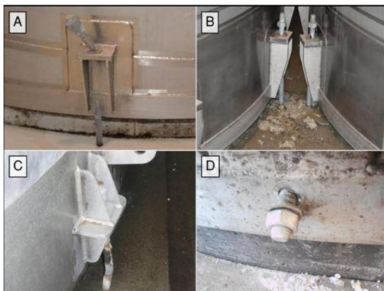
Figure 2-30: (A) Anchor rod tearing; (B) Pull-out of the anchor bolt; (C) Buckling of the anchor rod; (D) Pull-out of the anchor bolt (Rosewitz & Kahanek, 2017)
