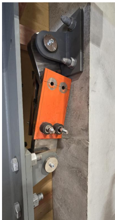
Figure 5-29: RSFJ with Ruptured Rods
