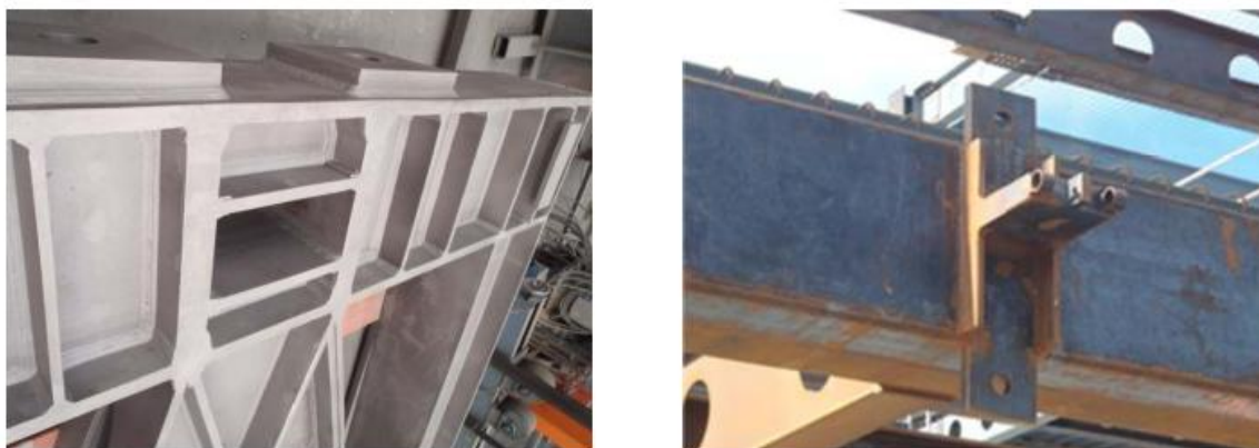
Figure 5-31: Seismic frame collector beam with slot for tongue plates (Latham et al. [2013])
