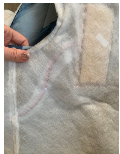
f) Fixing the covered components of the system to the insulation layer
