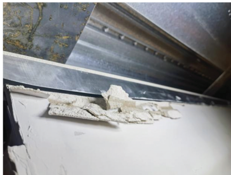
(b) Localised plasterboard damage with spalling and detachment (2.12%)
