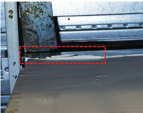
(a) Scraping off the plasterboard and deformation of the top DST flange (1.49%)
