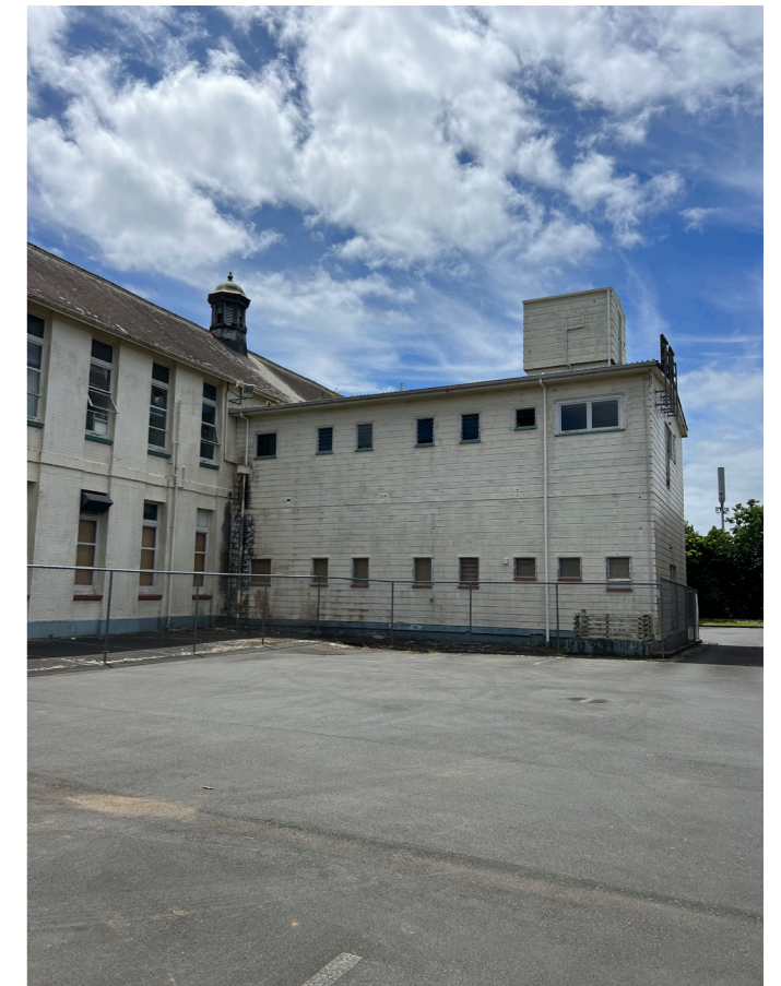
Figure 12 View of Building 5 1970s addition (Eastern Wing) looking Northwest. The cladding contains asbestos, the window openings are very small and do not relate to the original building. The junction between the addition and principal form roof is complicated.
