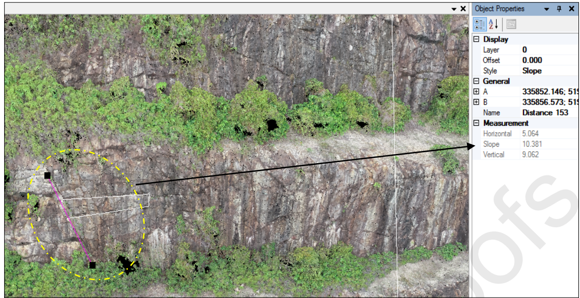
Figure 14: Persistence of the joint (purple line) measured is 10.3m.
