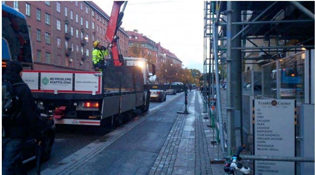
Figure 27 - Construction hazard example provided in the international literature (Niska & Eriksson, 2014)
