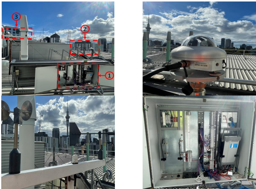
Figure 18: Location of solar still measurement sensors, 1: Data logger, 2: Anemometer,
