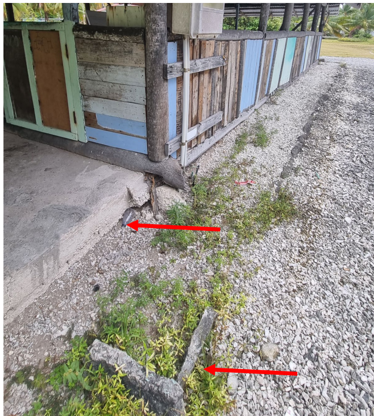
Figure 33: Old platform stones 1979 to perimeter of building. Interior replaced with concrete slab
