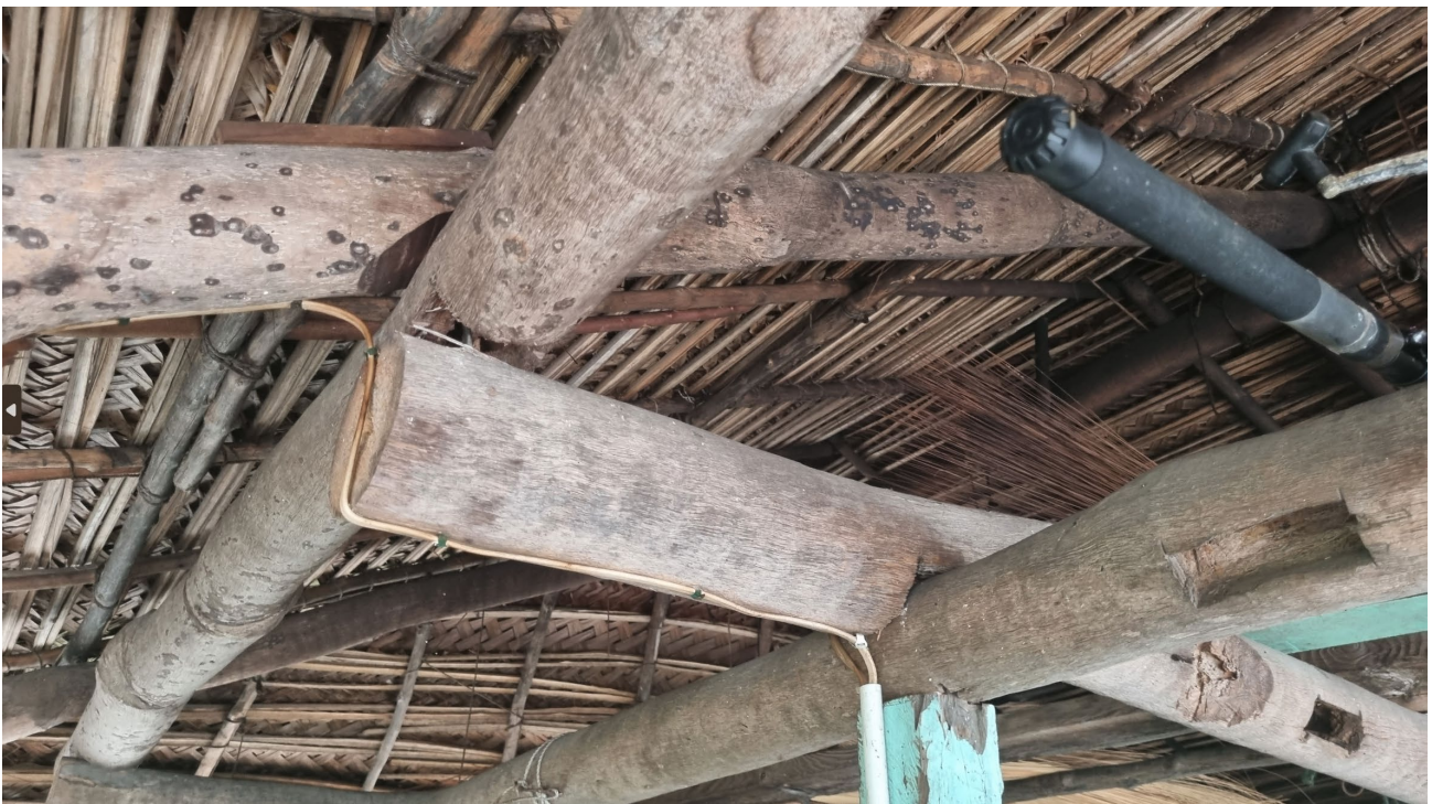
Figure 46: Underside view of post beam, rafter eaves connection. Note recycled notched wall plate
