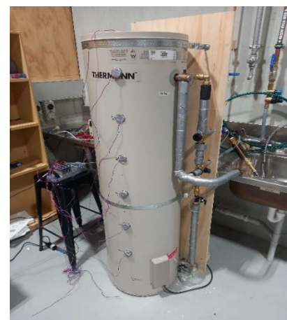
Fig. 23. Hot water cylinder setup showing sealed thermocouple plugs.
