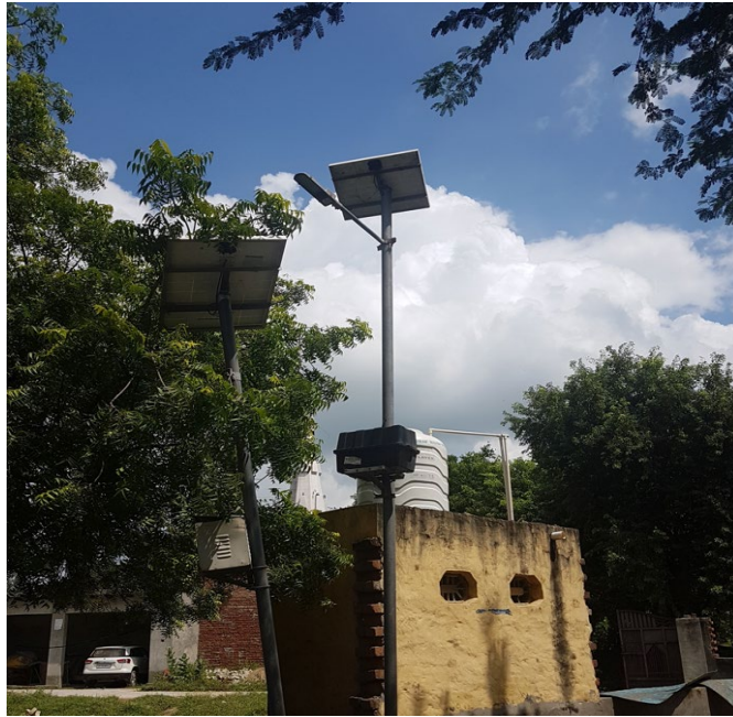
Figure 4-9. Solar Street Lights in Balanpur
