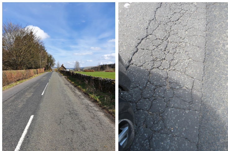
(a) Moderate Alligator Crack (b) Severe Alligator Crack
