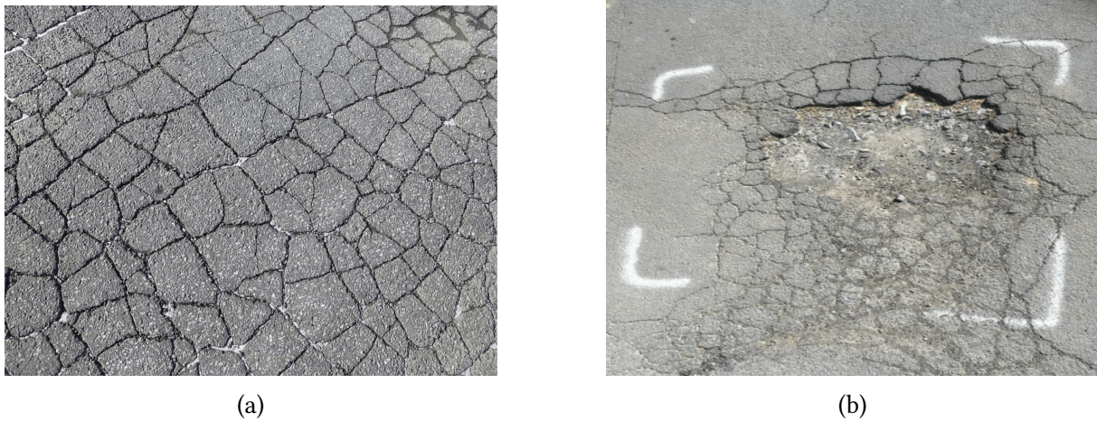
Figure 1.1: Examples of severe pavement deterioration resulting from neglected cracks [1].
