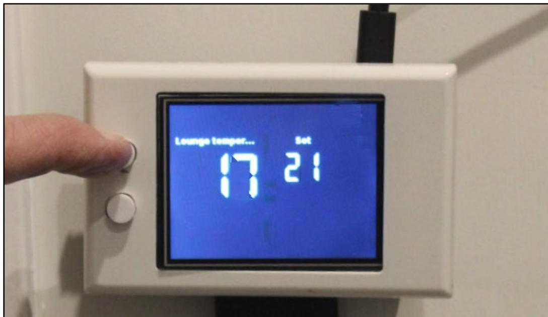
Figure 9.20: The HVAC room controller during a Stage 8 field trial.
