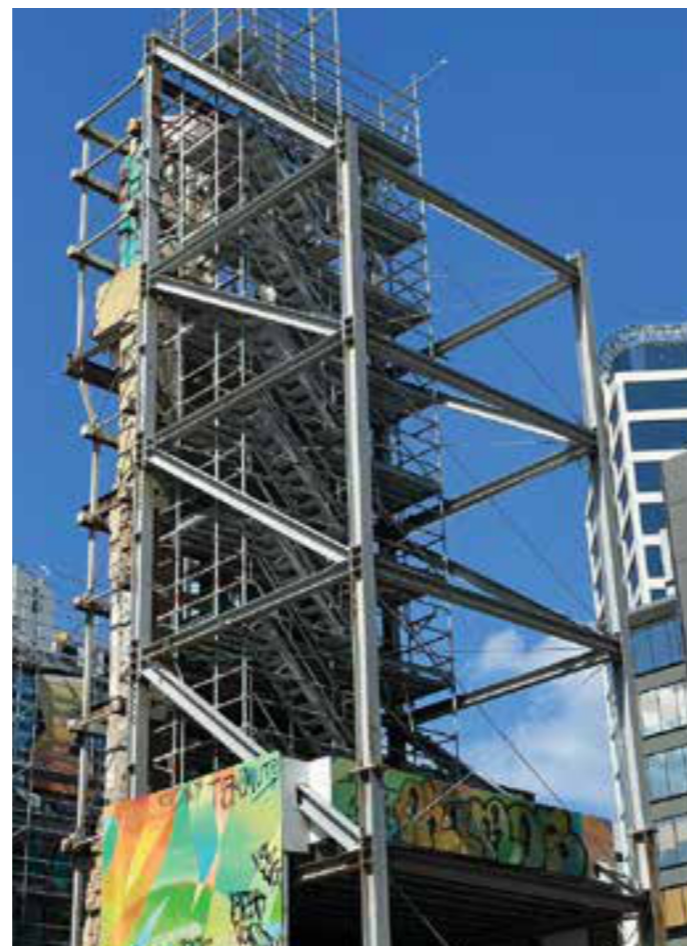
Figure 50. Looking up at the steel structure supporting the heritage facade from Queens Street. 2025
