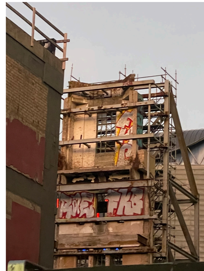
Figure 58. View of the St James Theatre heritage façade and temporary steel support structure from Lorne Street, 2025.
