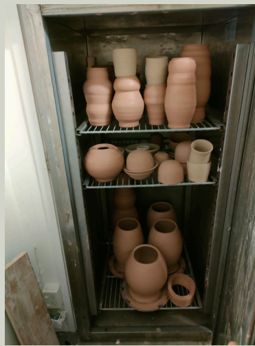
Broken Freezer View 16 th March 2023
