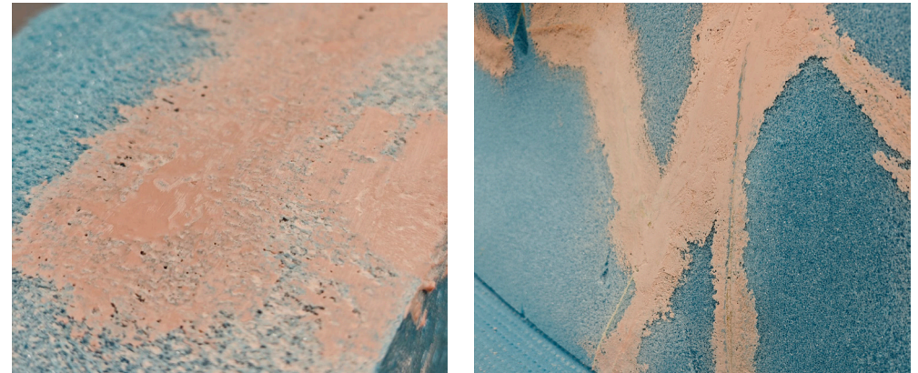
Figure 41. Wall filler covering the defect, Luwen Xu (Annie), AUT, 2026.
