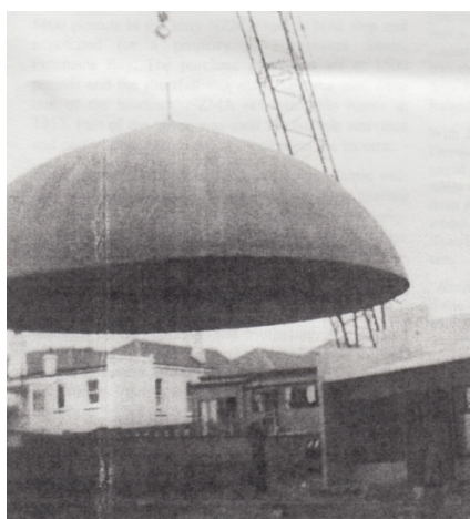
Figure 8. Steel dome for the Ponsonby Mosque being lifted into place, Tāmaki Makaurau Auckland, ca. 1979. Courtesy of the New Zealand Muslim Association. Reproduced with permission.
