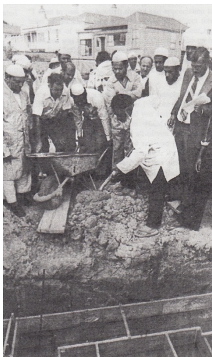
Figure 7. Suliman Ismail Bhikoo, first elect Chairman of the Ponsonby Mosque, places the first shovel of concrete for the foundations of the first masjid /mosque in Aotearoa New Zealand, Tāmaki Makaurau Auckland, ca. 1979. Courtesy of the New Zealand Muslim Association, reproduced with permission.
