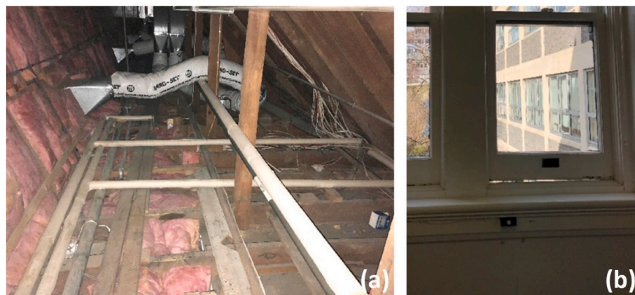
Fig. 4. Photos of case study C showing key issues. Photo credit: Priscila Besen.
