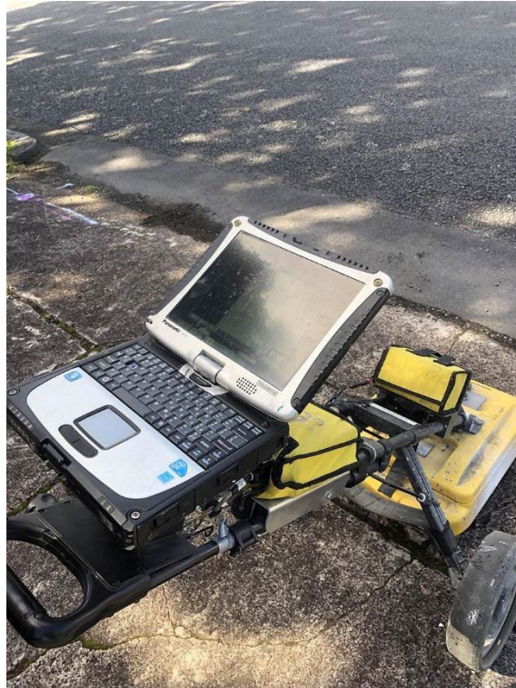
Figure 2-1 Ground-penetrating radar was used to identify the subterranean earth connection within a power station. The photos were taken by the author in 2017.
