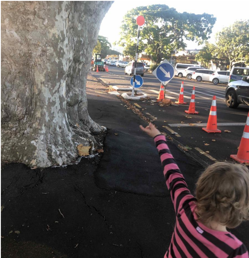
Figure 24: Tree and narrow footpath damaged by the roots; photo contributed by Lenny
